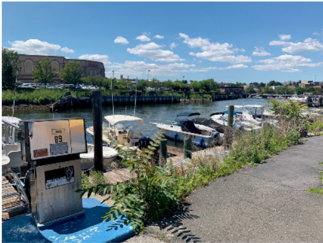
Commercial Gas Pump
